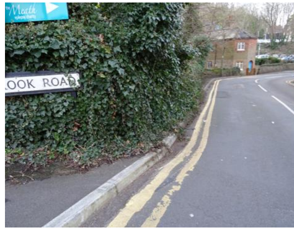
Footway submerged under vegetation
