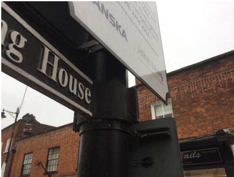
16a. Fingerpost High Street near Red Lion detail showing correct clamp fitting on a lamp column
