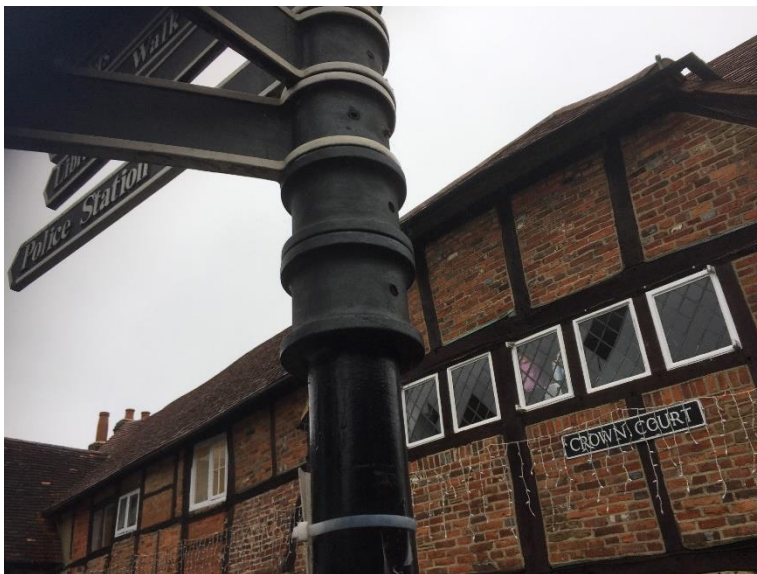
12a. Fingerposts in Crown Court/High Street detail showing that incorrect fittings have been used on a lamp column
