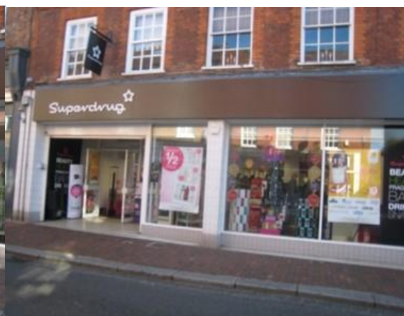
The one above has used glazed ceramic tiles and large plate glass which is a bland expanse out of character with the street
