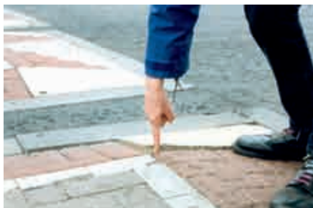
Fig. 2.8 Damage to a speed cushion
