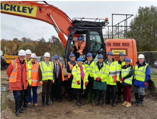
Jeremy Hunt MP in the digger with the Environment Agency project team and members of the partnership who have supported the project
