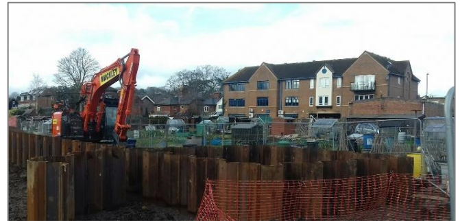
Sheet pile wall in allotments (before cladding). The square piling separate to the wall is for installation of the pumping station.
